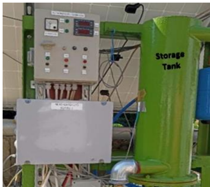
Figure 4. Arduino-based control unit and the storage tank
